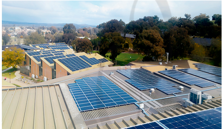
Figure 4-45 Roof PV in Australia
