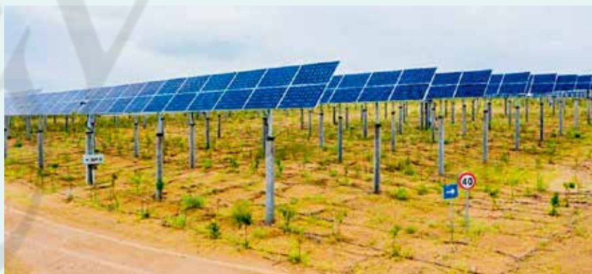
Fig. 1 Kubuqi Desert PV Project in Inner Mongolia, China
