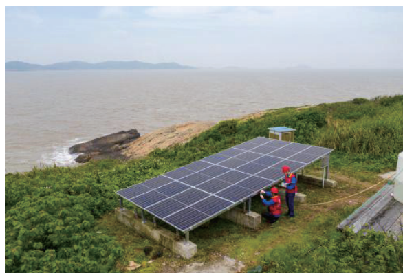
Donation for building zero-carbon micro-grid in the breeding ground of Chinese crested terns in Xiangshan
