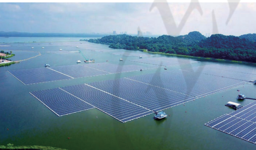
Singapore Tengeh Reservoir Floating Power Station Project by Sembcorp Industries
