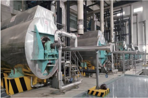
Sludge drying system
