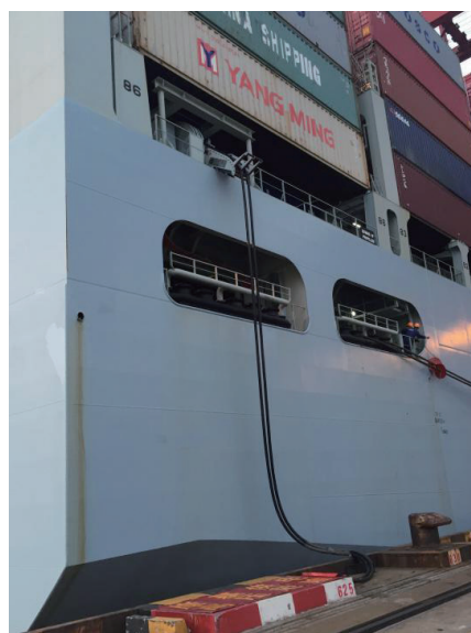
(b) COSCO Denmark connecting to shore power
