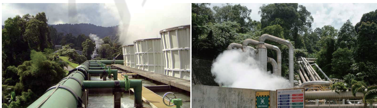
Gunung Salak geothermal power station facilities
